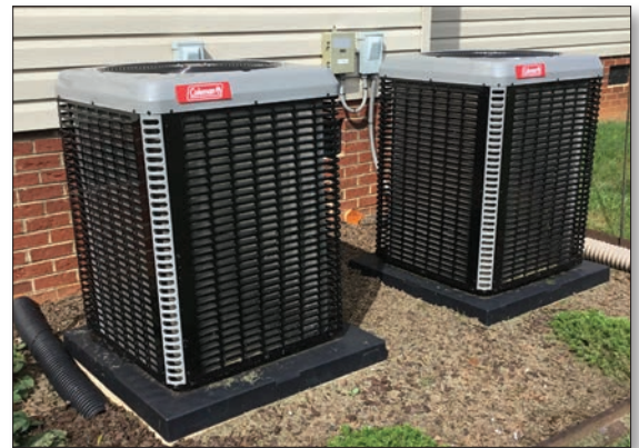
3-ton HVAC units
