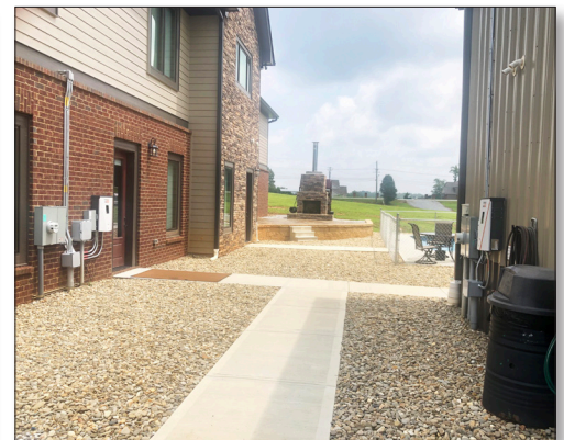
Install Involved 2 Power Meters 12' Apart
