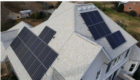
Solar panels can be placed on separate roof areas to face different directions or be ground mounted.
