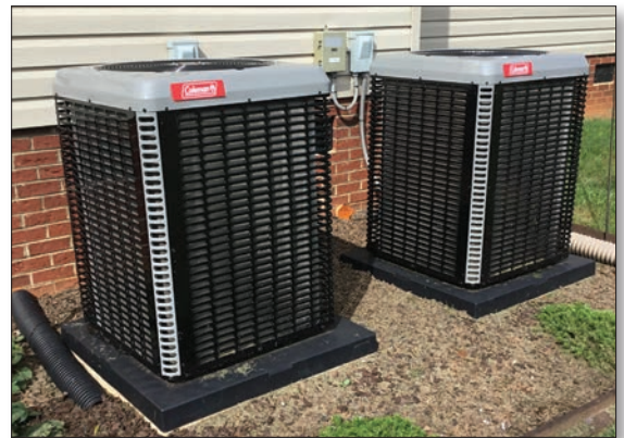
3-ton HVAC units
